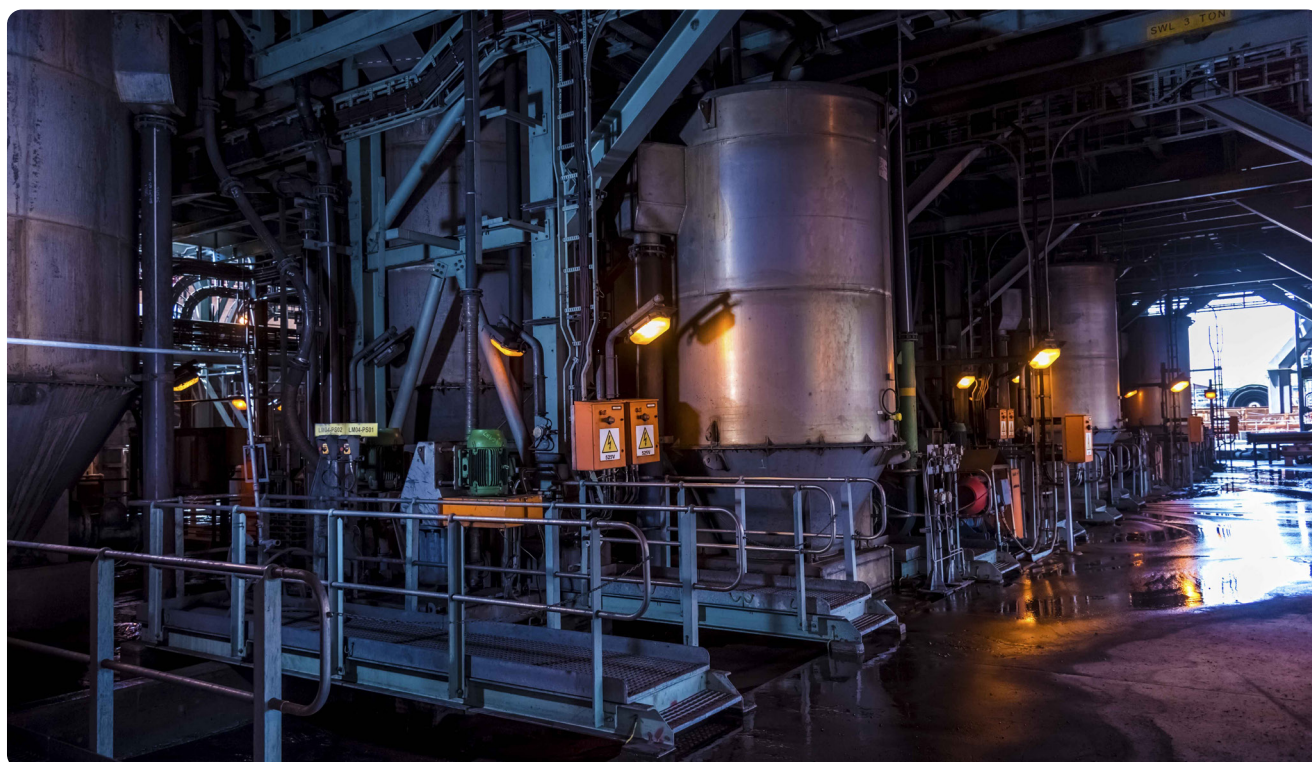
Inside a coal beneficiation plant at our Grootegeluk BU
