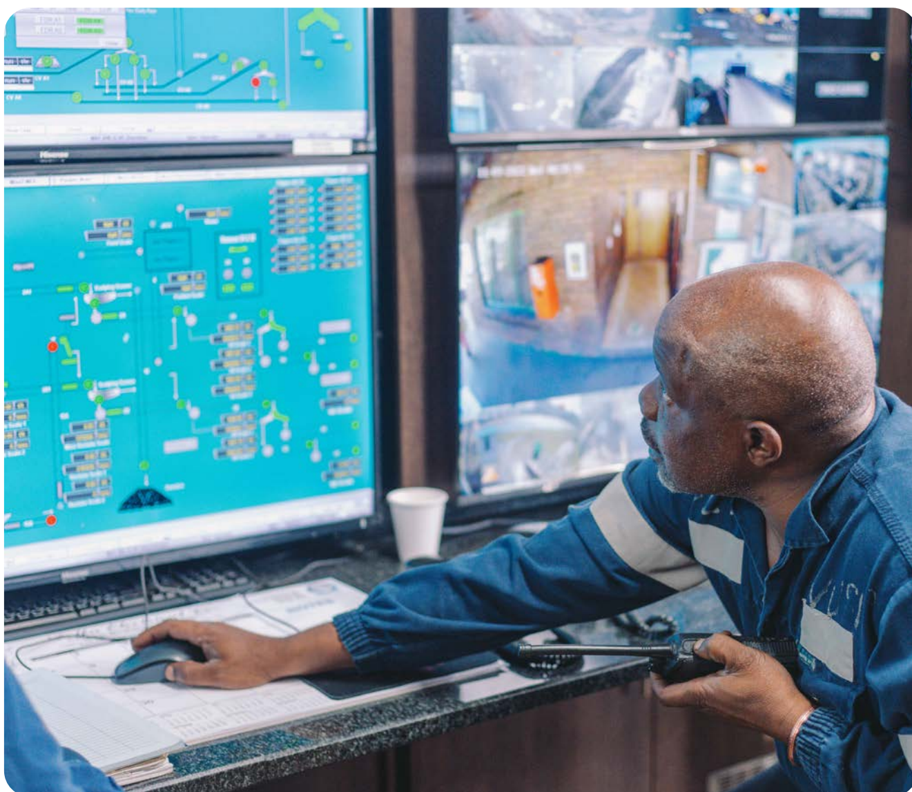
Matla control room
