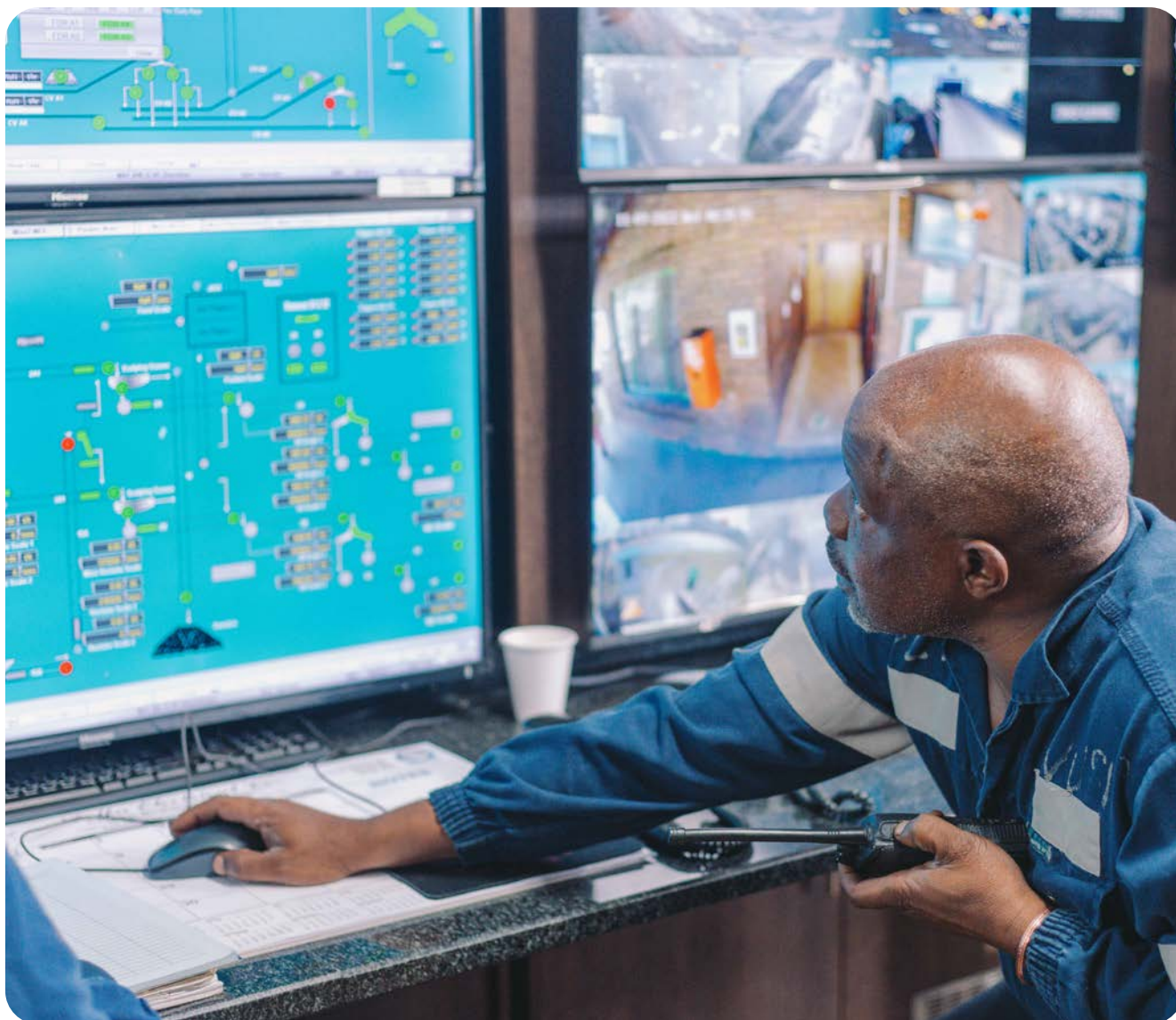
Matla control room
